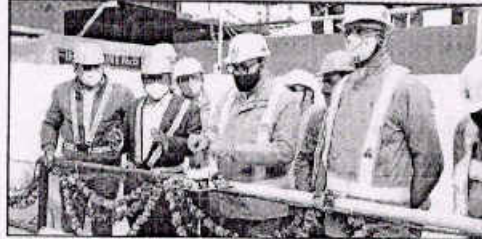
October last year. The tunneling has started from the Vikaspuri station in the eastern part of the city. The drive is being undertaken by the DMRC's Managing Director, Dr. Manoj Singh and other senior officials.
