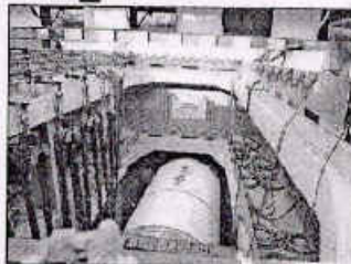
The tunnel will be built up with proven technology of EPBM (Earth Pressure Balancing) method with cutting tools made up of premium quality steel. The tunneling drive is being undertaken by the DMRC's Managing Director, Dr. Manoj Singh and other senior officials.
